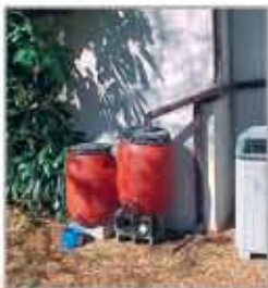
Gutters and downspouts funnel rainwater to the rain barrels.
